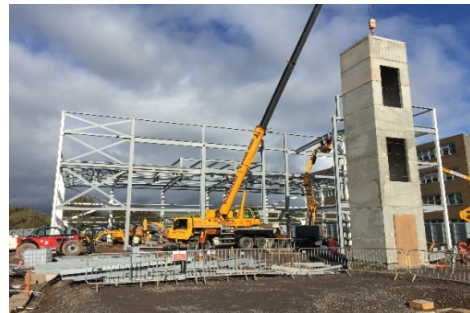
4 Sports Hall and start of steel frame of main school building with Lift Shaft No. 1
